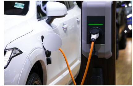
81 - Electric vehicle charging
